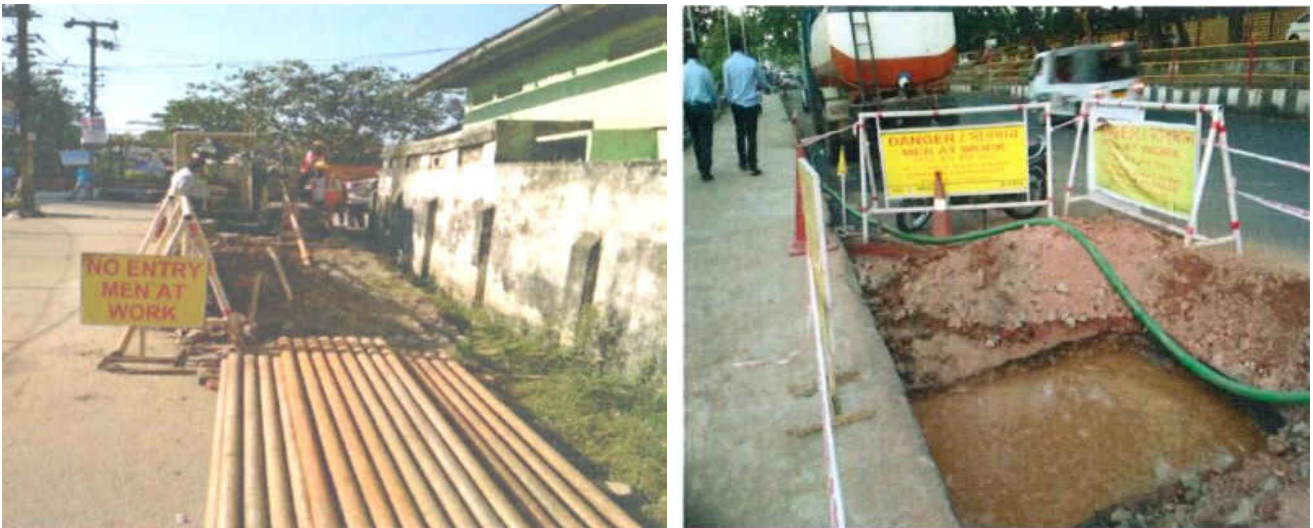
Proper Barricading of Work Area
