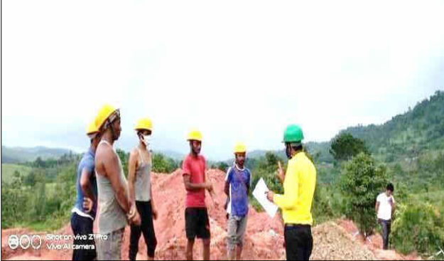
Safety briefing on Excavation, First aid, PPEs in 220 kV D/c Byrnihat-Mawngap-New Shillong
